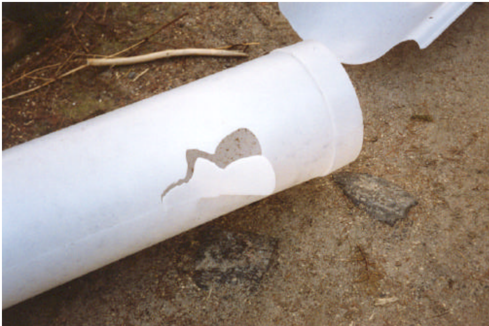
Plate 6 Damaged Section at the Road
